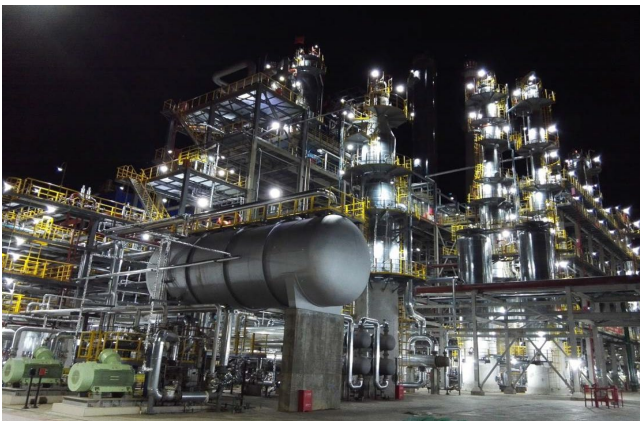
petrochemical device and other hazardous places
