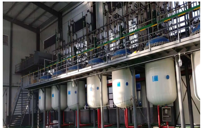
workshop and equipment area of pharmaceutical and chemical enterprises
