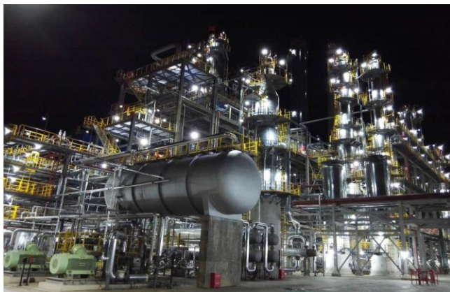
petrochemical device and other hazardous places
