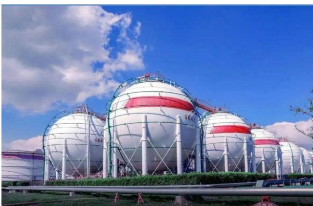
oil depot and chemical tank area
